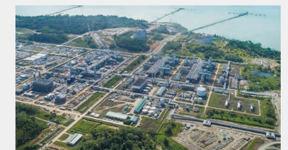
Liquefaction plant existing second system and expanded system under construction, LNG tanks, jetty, etc.
