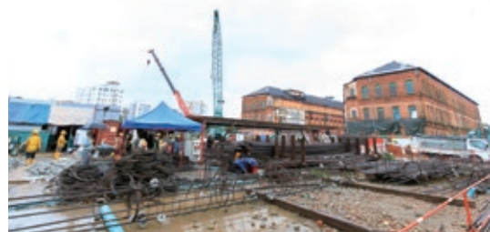
As Yangon experiences a long rainy season, work interruption due to downpours happens almost daily. Despite such bad conditions, the construction is progressing safely and on schedule based on the plans
